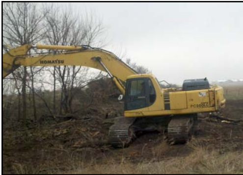
An excavator clears the site for the first phase of the North Dry Creek Streamflow Augmentation Project.
