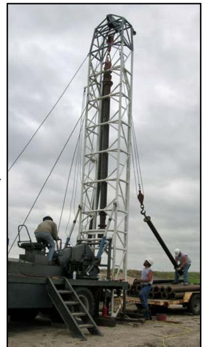
A crew from Holdrege Well Service drills the first well for the streamflow augmentation project.
